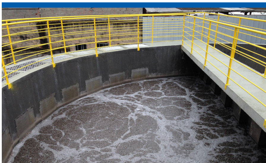
Biowater's CMFF Process after UASB reactors.
