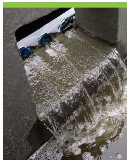
Secondary clarifier effluent.
